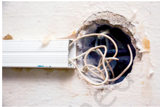
Fig. 1.28: Be careful of exposed cables
