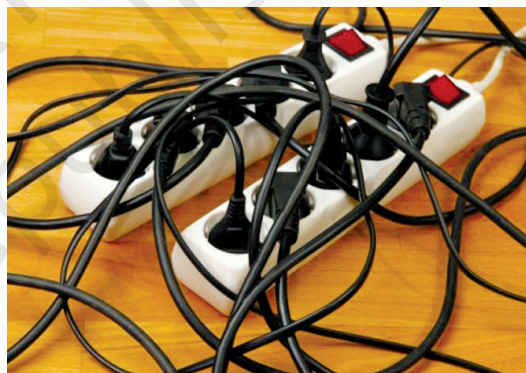
Fig. 1.29: Overloaded extension cords
