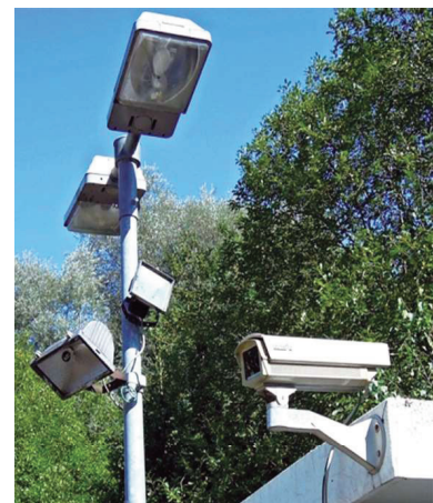
Fig. 3.9: Security lighting system with CCTV camera
